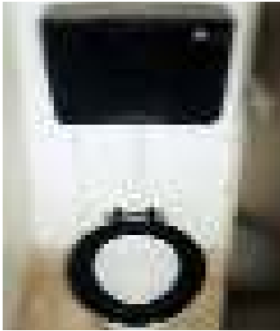
Old toilets before replacement
